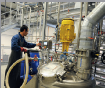
Mixing tank in Elven
